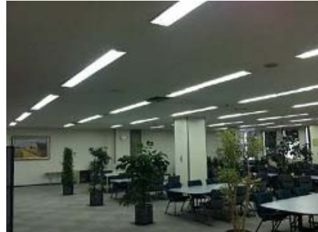
LED lighting in the Hamura R&D Center lobby
